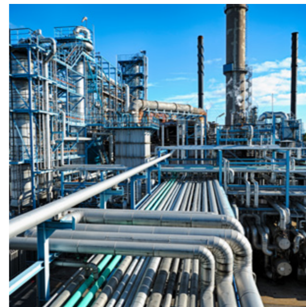
Oil Facility Canada
